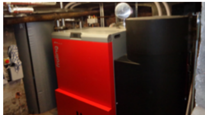
Figure 6 – Gwent Energy installed 100 kW biomass boiler at Wellington Baptist church and community centre (Gwent Energy CIC, 2019c)
