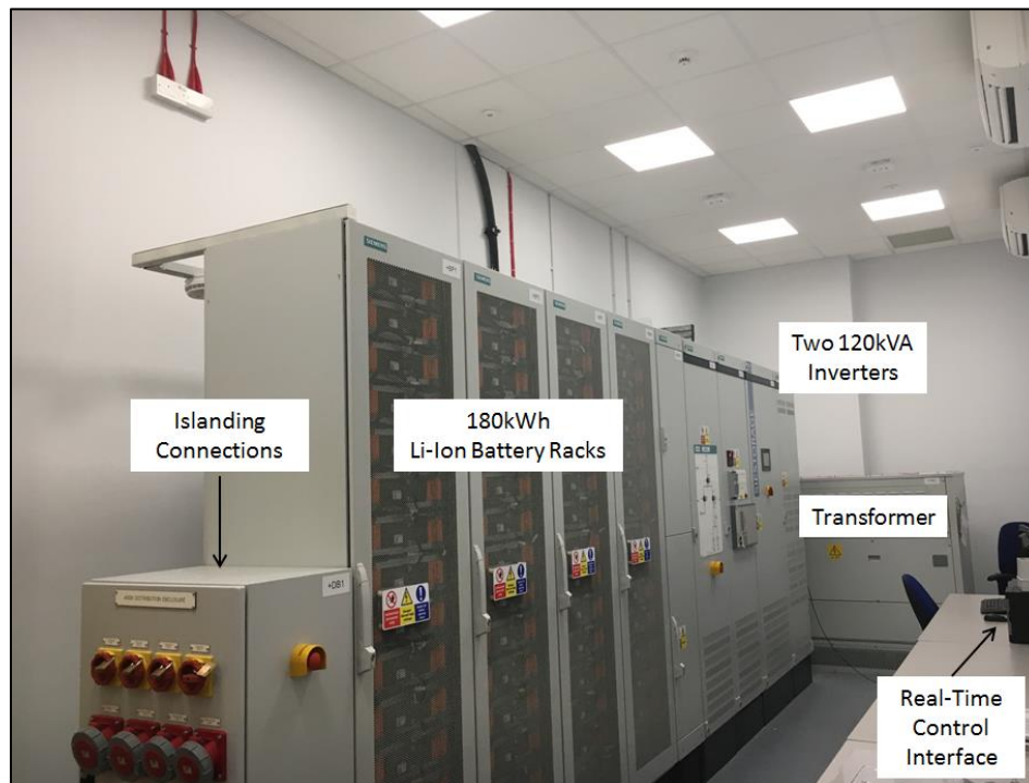
Fig. 2. The University of Manchester Energy Storage System
