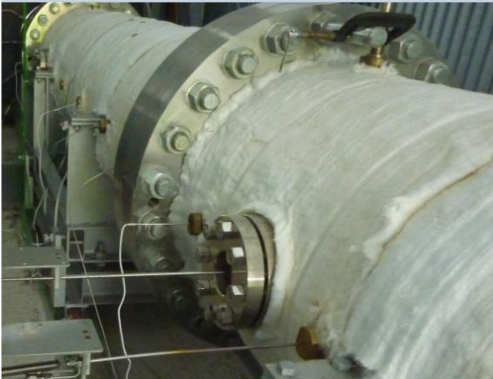
Figure 4: Circular duct sections with insulation
