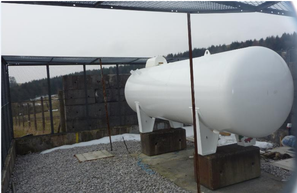
Figure 6: Butane supply tank
