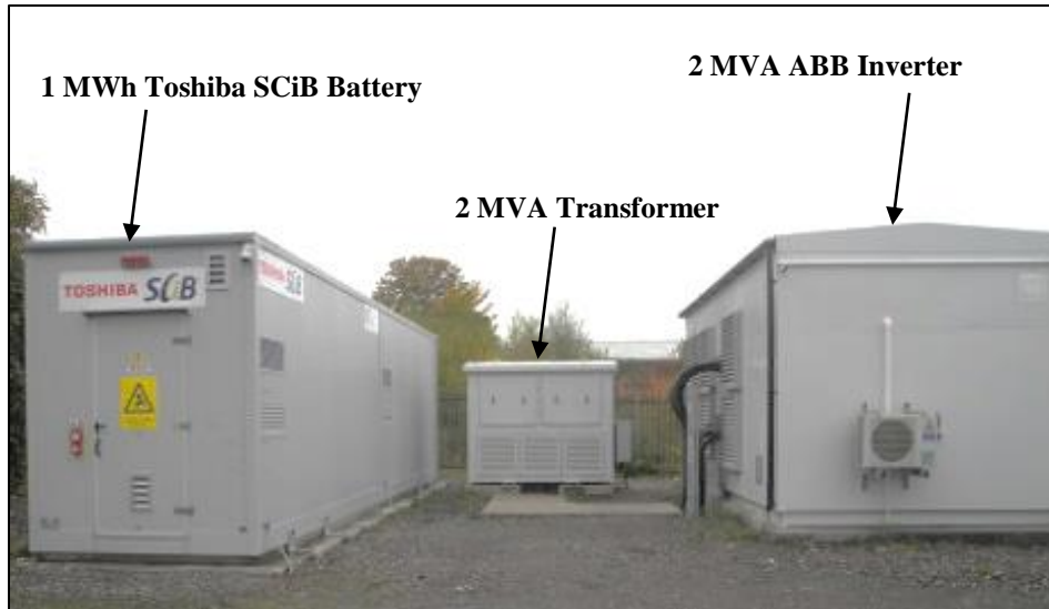
Fig. 1. The Willenhall Energy Storage System (WESS)
