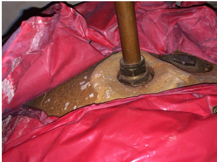
Figure 11 – No Immersion Heater
