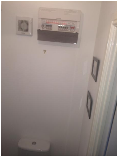
Figure 10 - Inappropriate location (customer toilet)
