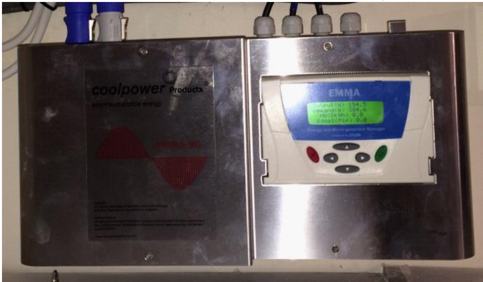
Figure 4 – EMMA RJ45 Connection point
