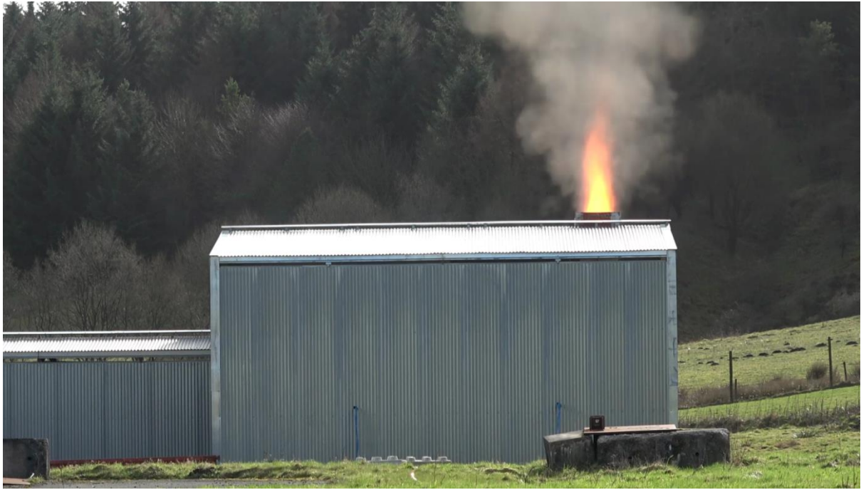
Figure 10 Flame emerging from the vertical chimney at the end of the HRSG.
